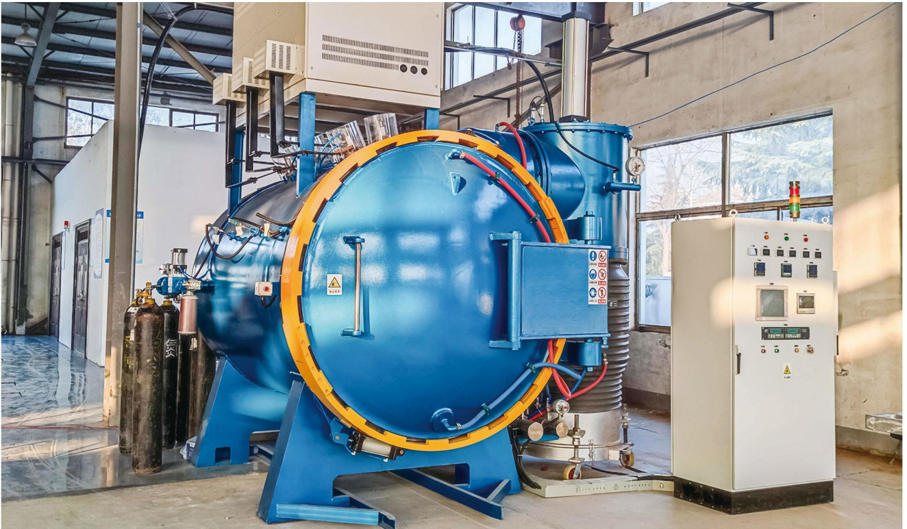
钎焊炉 Brazing furnace
